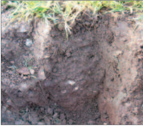
A compacted subsoil can lead to slow drainage.
